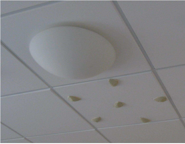
Figure 2: A six-element microphone array installed on the ceiling.
